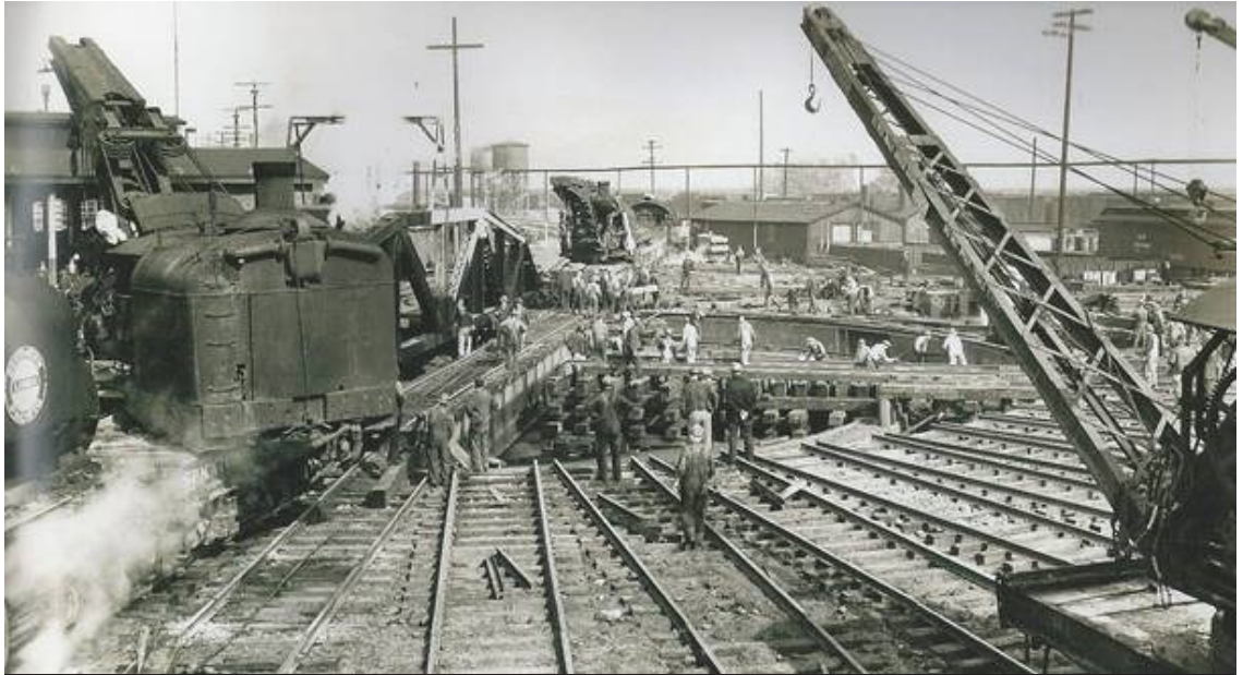
Southern Pacific Crews work to complete the installation of a new 110-foot turntable at Bayshore (San Francisco) in 1941. Southern Pacific Railway pic.
